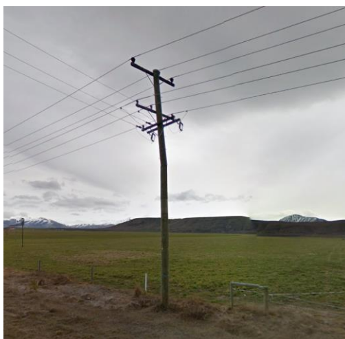
Figure 3 - A typical pole on the Twizel to Omarama line, showing 33kV over 11kV construction
